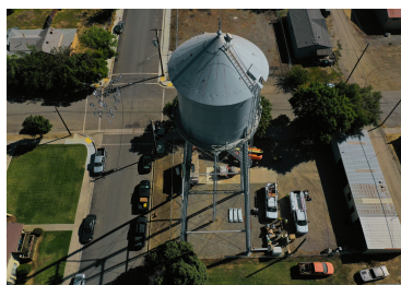
Maxwell Water Tower Railing - 4 Radios
