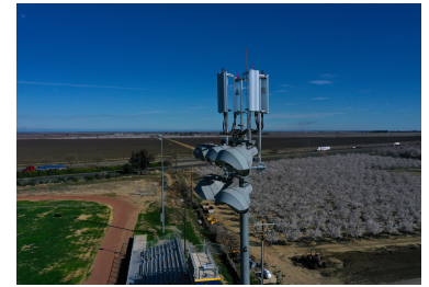
Pierce HS Football Field Light Pole - 4 Radios
